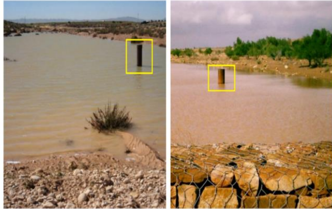
Recharge wells installed in the study area behind a gabion check dam injecting floodwater after a rainstorm
